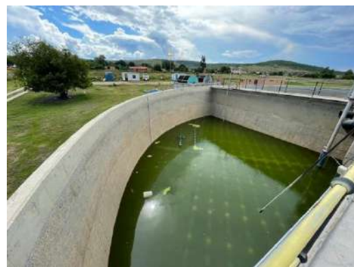
Photo 6.6. Sewage plant in Swartruggens, built in 2012, which is in a state of disrepair.
